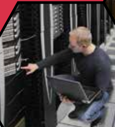
ITMAX DATA CENTER SOLUTION
